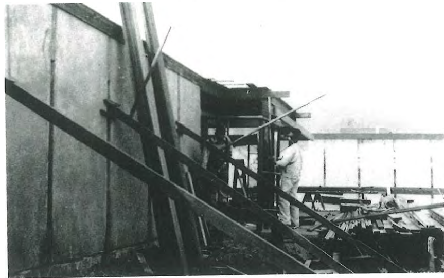
Building the redwood framing and roof on the Marian Chace studio, ca. April 6–24, 1922
