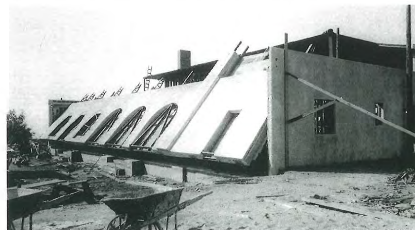
Irving Gill, La Jolla Woman's Club, La Jolla, California, 1913. The club was built using the tilt-slab construction method
