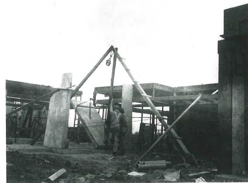
Tilting a slab into place with the block and tackle, ca. March 28–April 24, 1922
