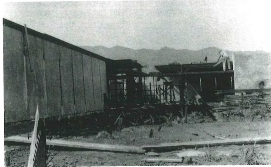
Building the redwood framing and roof on the Clyde Chace studio, ca. April 24-May 1, 1922
